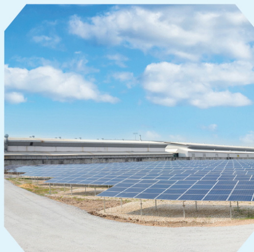
3.35 MW Bangbuathong Agricultural Cooperative, Ltd.
